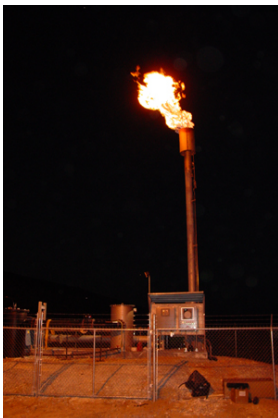
Flaring of landfill gas
