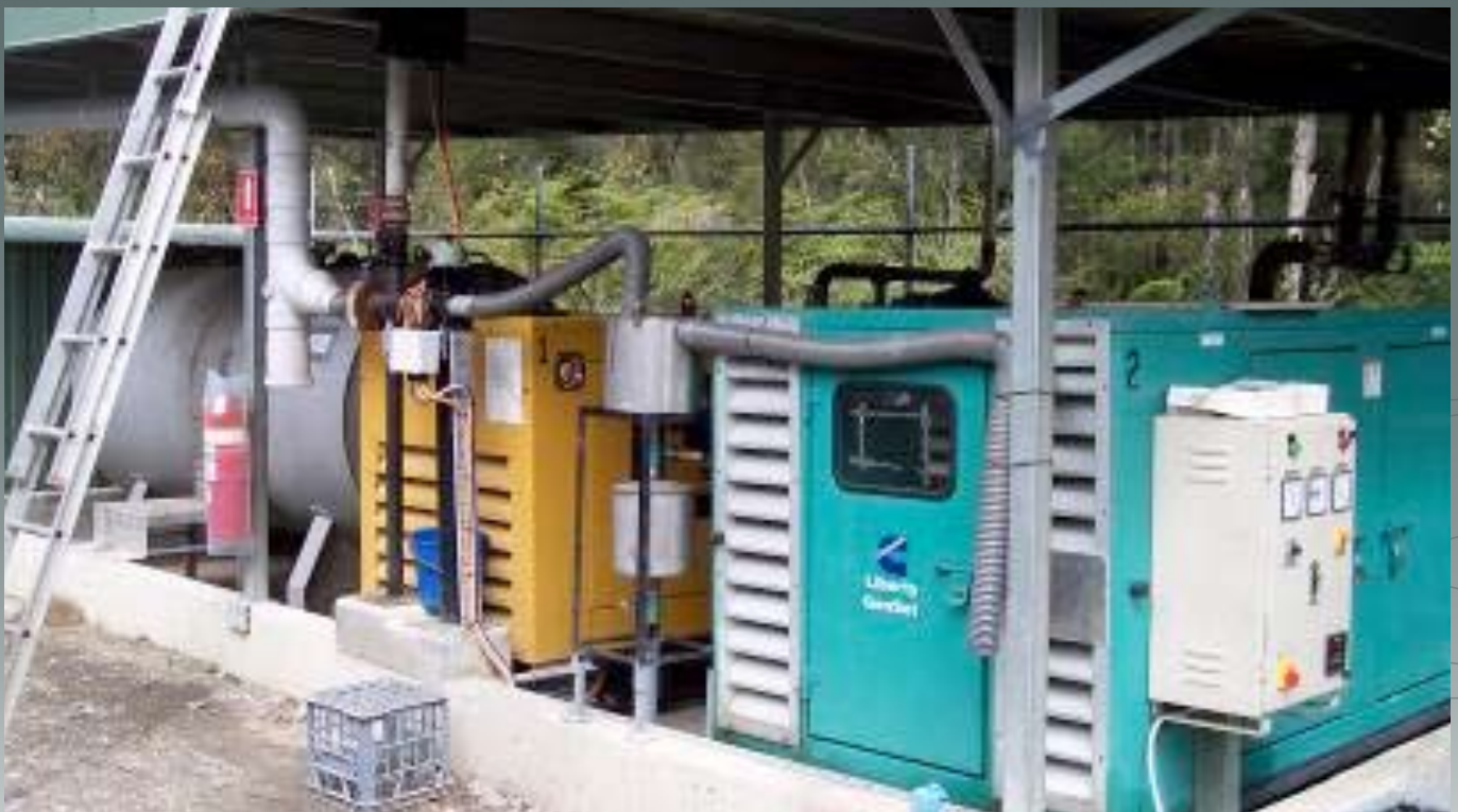
Figure 5.2 : Dual Fuelled Generator Set Coupled to Ankur Gasifier
