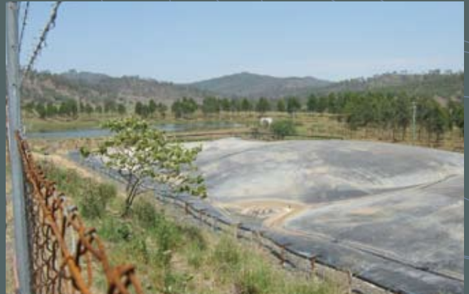
Figure 2.10: AJ Bush Digester at Rendering Plant
