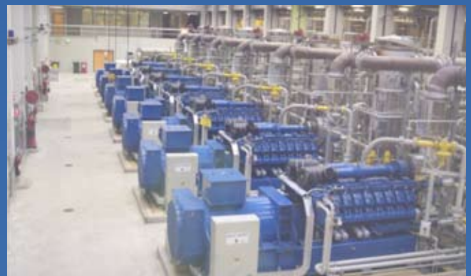
Figure 2.7: Carrum Downs Generation Hall
