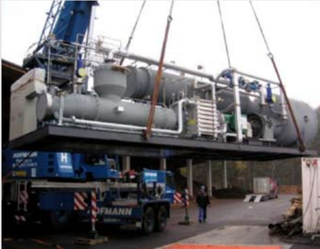
Figure 5.4: ORC Unit at Oerlinghausen-D -600 kWe
