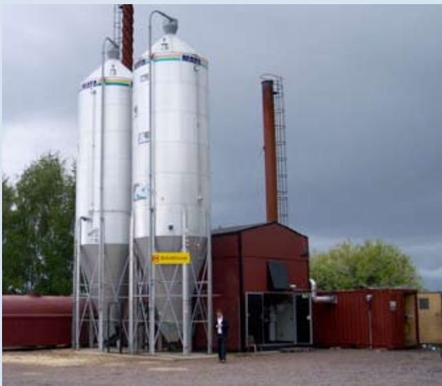
Figure 3.5: Wood Pellet Fuelled Central Heating Plant in Sweden
