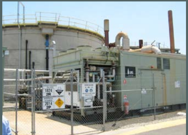
Figure 2.11: Oxley Creek Digester and Generator Set
