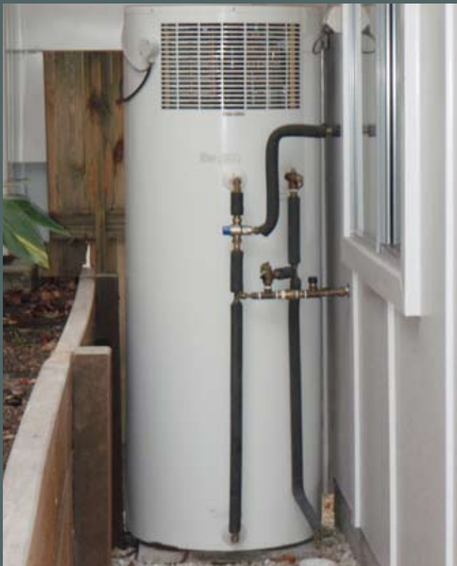
Figure 3a: Heat Pump installation
